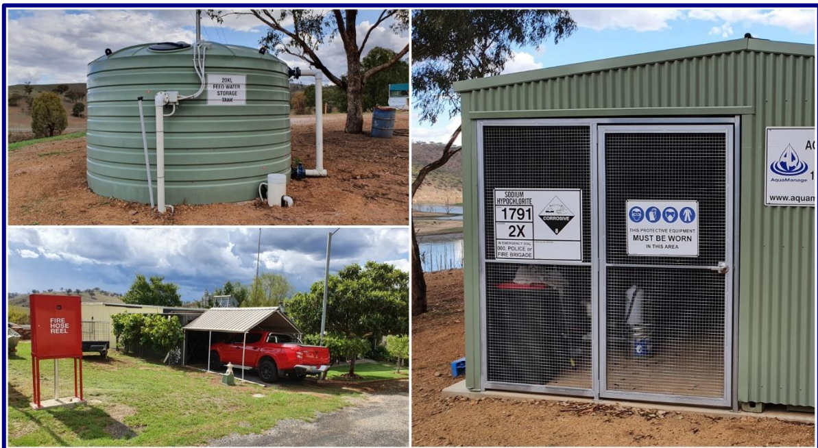
Figure 19 – Assets Holiday Park: Water Infrastructure Top LHS clockwise: Water treatment plant; fire hydrant.
