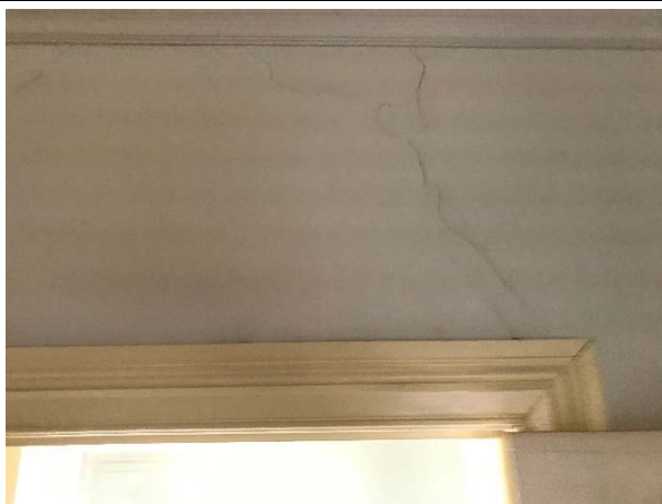
Figure 2 – Cracks in render, 2mm approx. generally throughout
