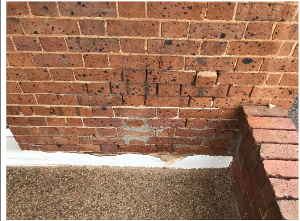
Figure 13 – Rising damp and failed mortar
