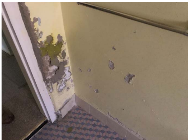
Figure 8 – Spalling render and rising dam, throughout
