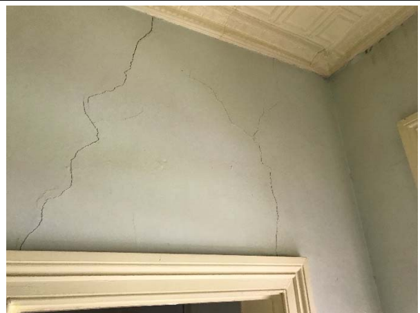
Figure 3 – Cracks in render, 2mm approx. generally throughout
