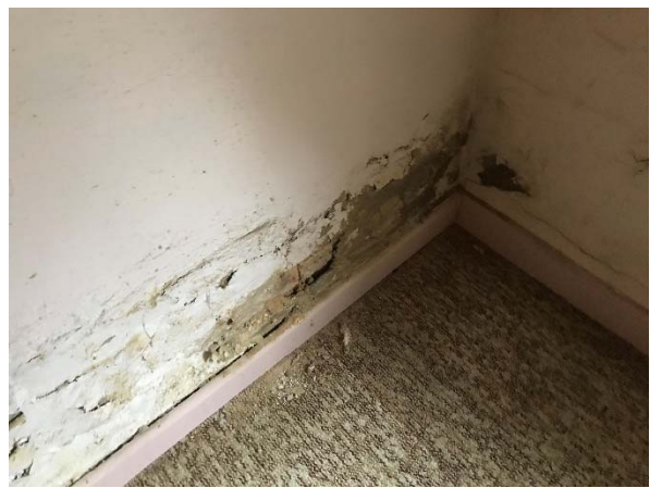
Figure 10 – Spalling render, mortar failure and rising dam, throughout
