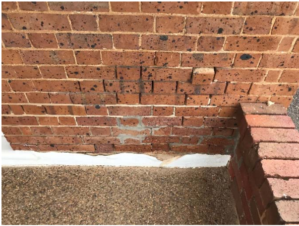
Figure 12 – Rising damp and failed mortar
