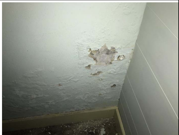
Figure 7 – Spalling render and rising dam, throughout
