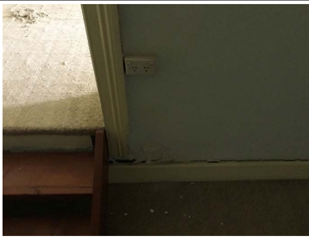
Figure 6 – Spalling render, rising dam, detached skirting and failed flooring sections throughout
