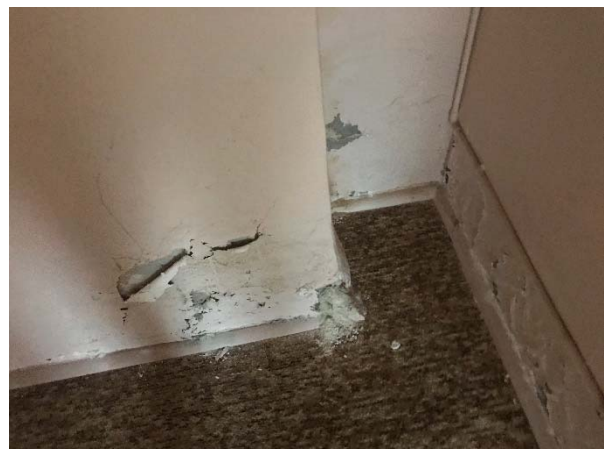
Figure 11 – Spalling render, mortar failure and rising dam, throughout
