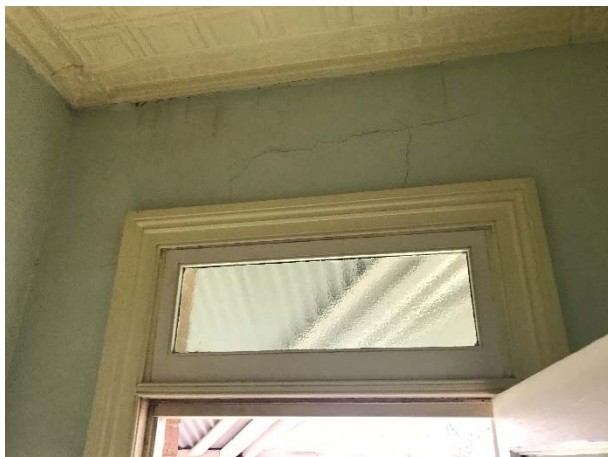
Figure 4 – Cracks in render, 2mm approx. generally throughout
