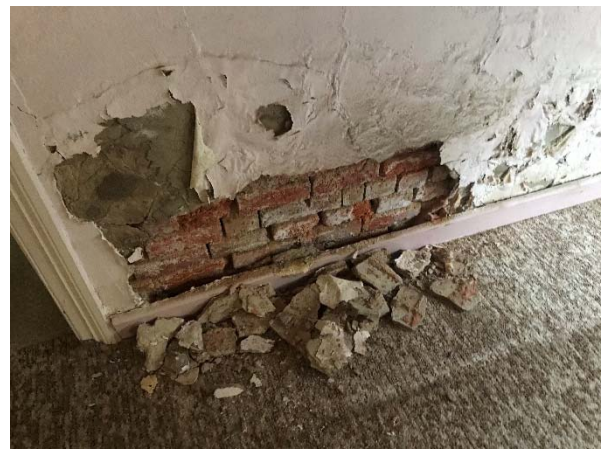
Figure 9 – Spalling render, mortar failure and rising dam, throughout
