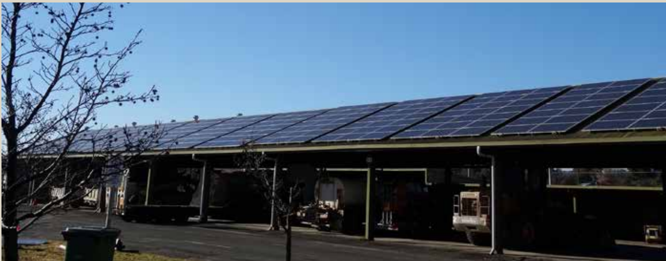
Solar panels on Council depot. (L. Hall)
